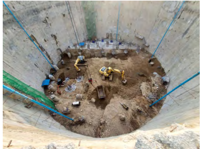
CAMANA Water Reclamation Facility (2022)
