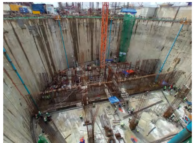
CAMANA Water Reclamation Facility (2022)
